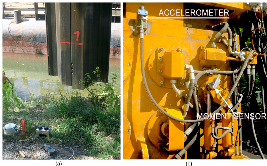
Fig. 3. Installation of double sheet pile in trial area; see Fig. 2: (a) view of geophones; and (b) instrumented vibrator.
